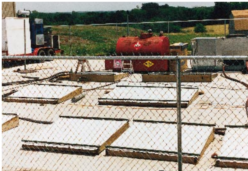
KWA's tank pits where the leak detectors are installed
